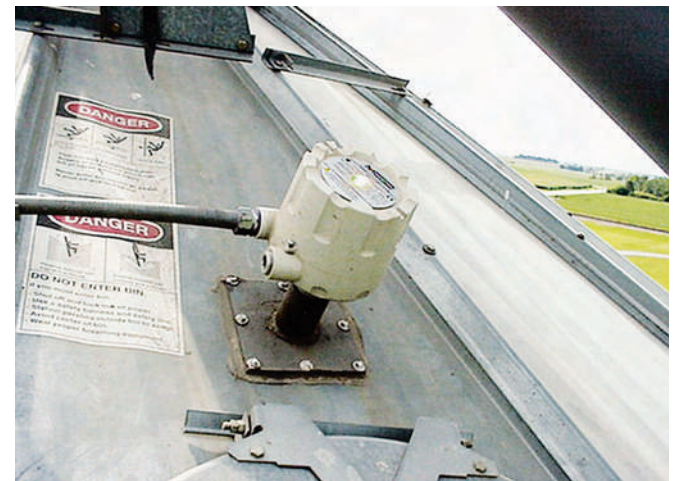
A self-validating point-level sensor on a grain bin
