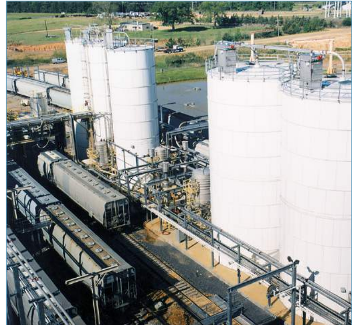
Railcar transfer to and from silos
