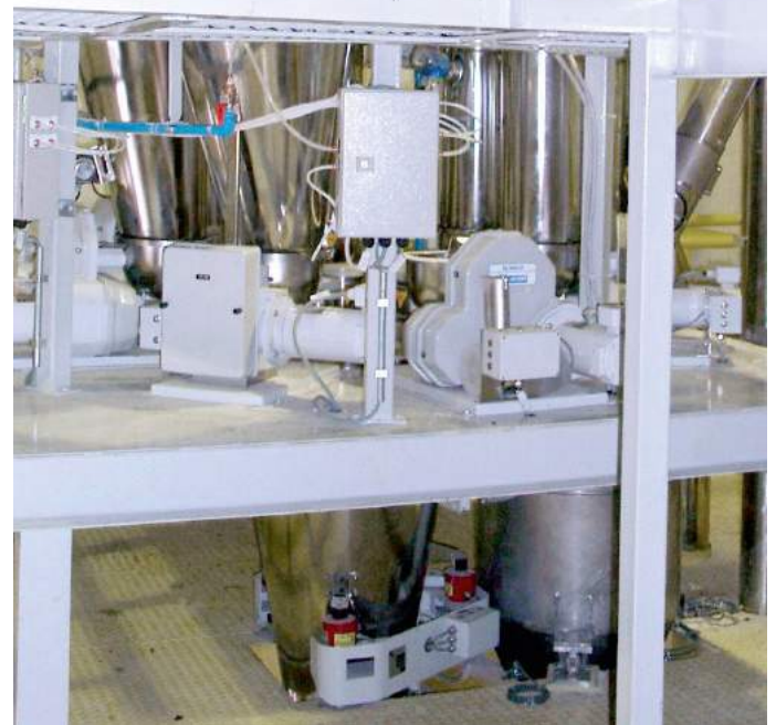
Gain-in-weight batching station for a bakery installation in Indonesia.
