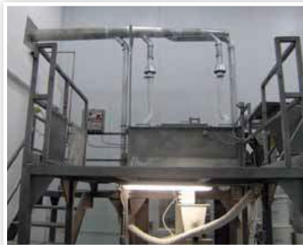
Stainless ducting is used with this dump station. Ducting is attached to DustHog SFC 32-4 above.
